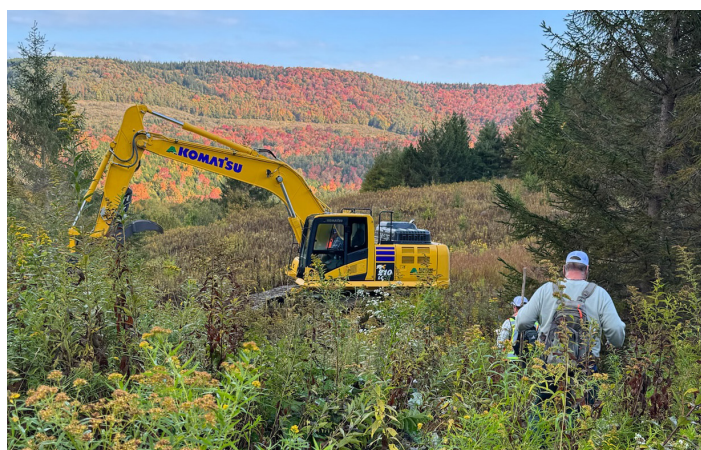
Contractors walk an excavator to the restoration area to begin pond decommissioning in fall of 2023.
